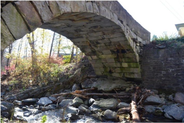
West Townshend Bridge needs repairs Photo by Andy Snelling
