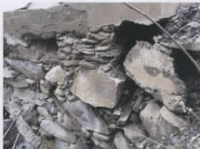
Collapsing section in northeast spandrel wall
